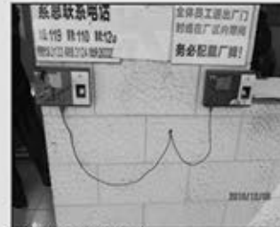
Photo of the sanitary facilities Attendance recording machine.JPG
